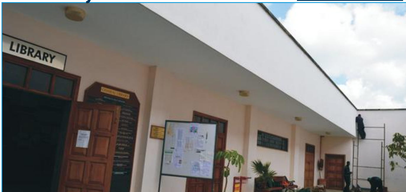
Previous view of the open space in the Library Verandah without a roof top
